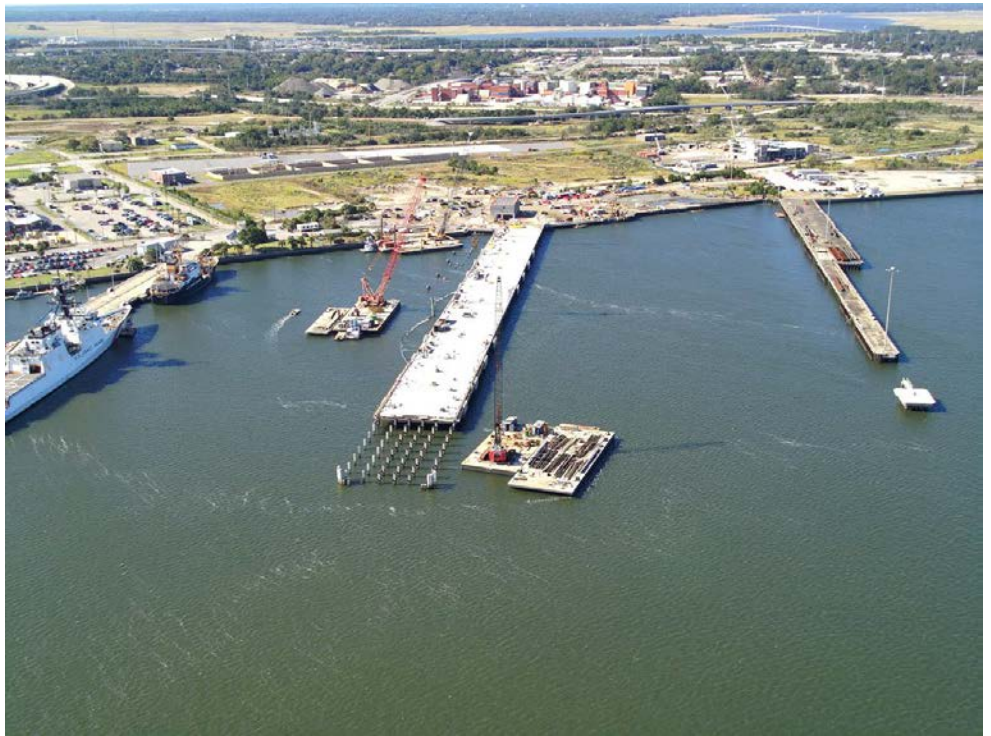
U.S. Coast Guard Base Charleston, South Carolina, Piers Papa, November, and Mike (left to right) showing work in November 2025, well advanced. Drone photo by USCG Base Charleston.
